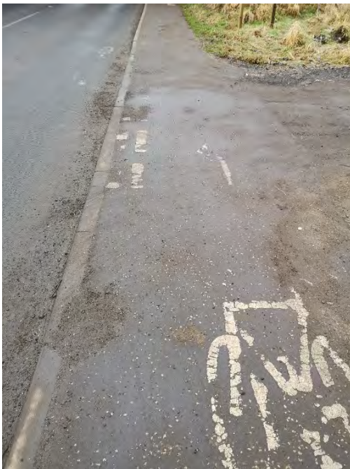
Figure 6 – Worn markings on B8000
